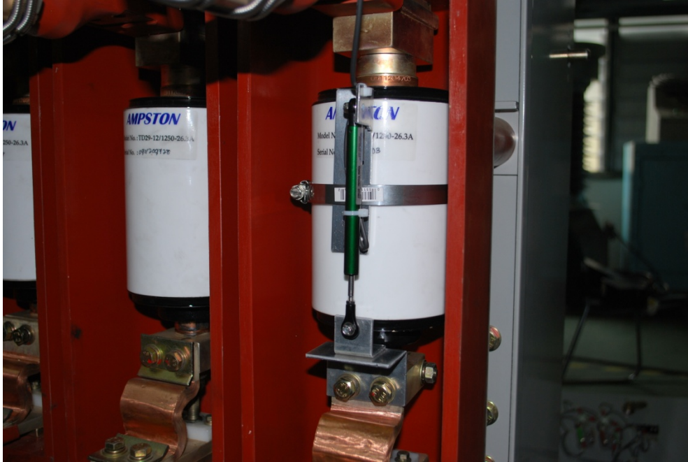
Resistor Transducer on Vacuum Circuit Breaker
