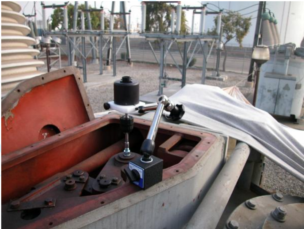
Rotary Transducer on Federal Pacific Circuit Breaker
