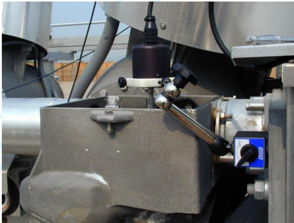
Rotary Transducer on Alstom HE 1014 Circuit Breaker
